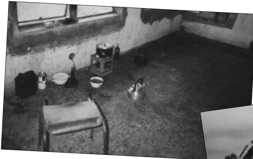
A dilapidated and now abandoned wing of the Gokana Hospital, Ogoni, Rivers State (left). (Photo: Alfredo Quarto)
